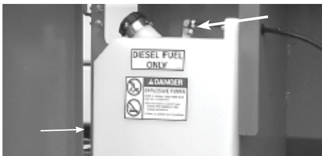
Figure 7.3 - Fuel Leaks at Tank
