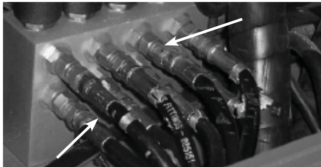
Figure 7.14 - Check Fittings at Valve
