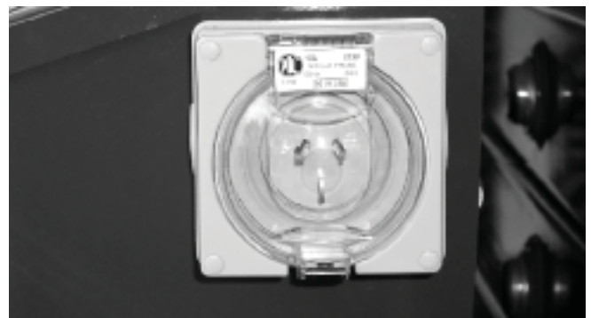
Figure 11.7 - Mains Power Connection For Charger
