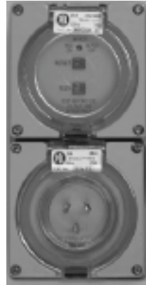
Figure 11.8 - RCD / ELCB Outlet
